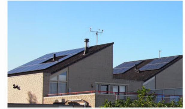
Roof solar system
