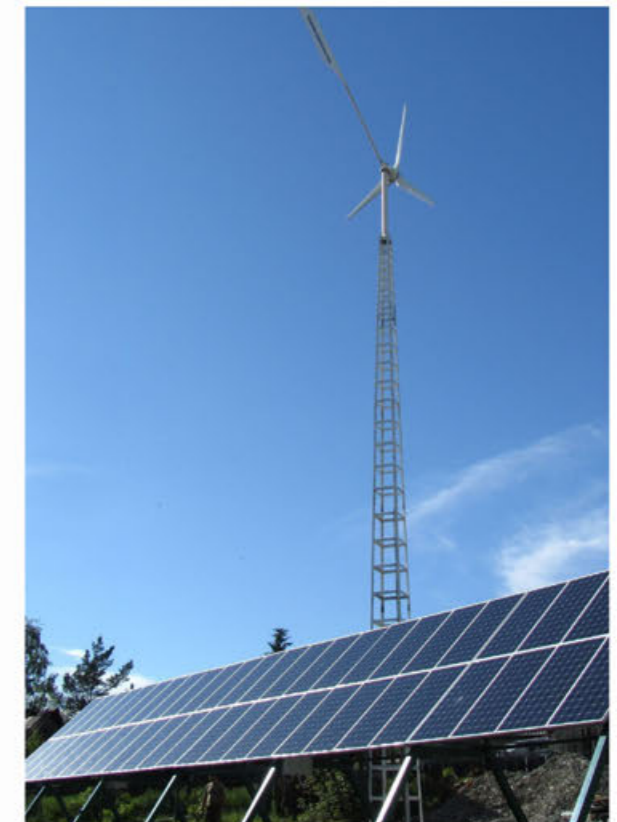
Telecommunication base stations solar system
